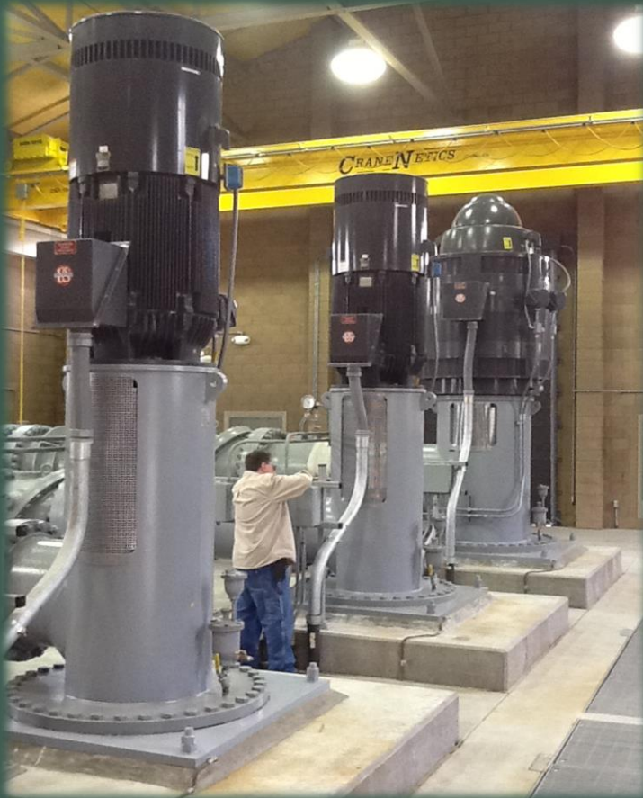
Grandsen Pump Station
