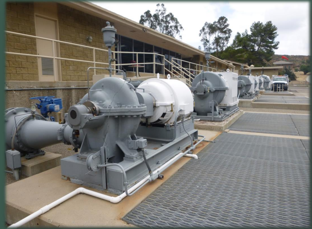
Conejo Pump Station
