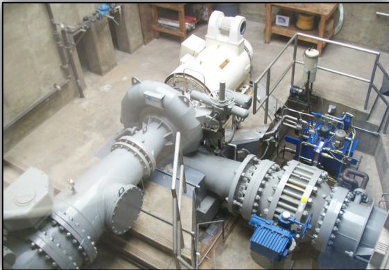
Springville Hydroelectric Generator
